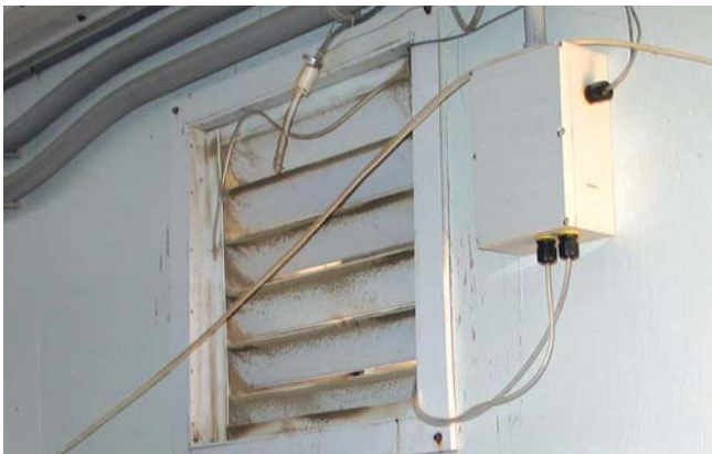
Air sampling equipment at barn ventilation points
